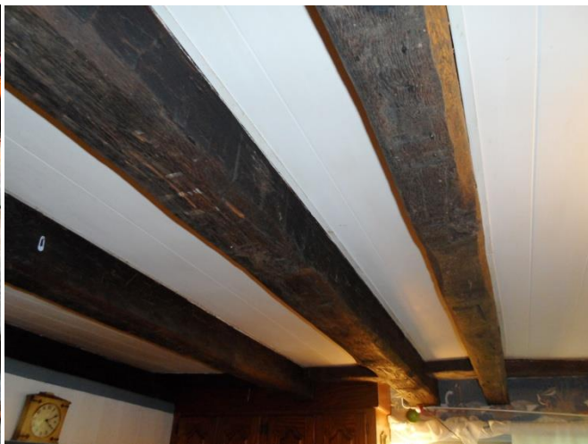
Left Above– well opening and cover in summer kitchen Right Above – beams in lower level kitchen and dining area which span the 30 foot space from north to south Left Below – hand hewn beam in unfinished basement area showing ax or adze marks, note subfloor is not whitewashed and is not original Right Below – multiple hand hewn pegs inserted in basement beams; likely used for hanging storage
